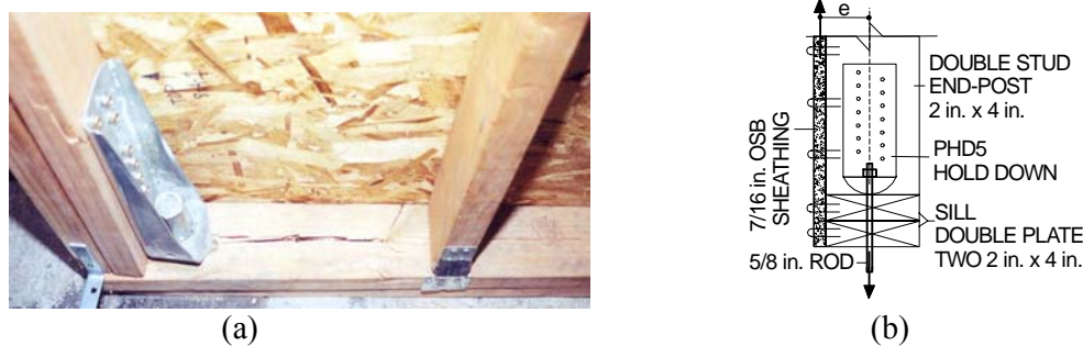
Figure 6. (a) Anchor rod failure and sill plate damage for panel 8-C; (b) hold-down detail.
