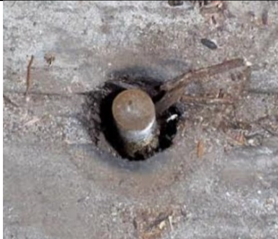
Hole in Mudsill is over ¼ inch in diameter. A gross violation of the building code
