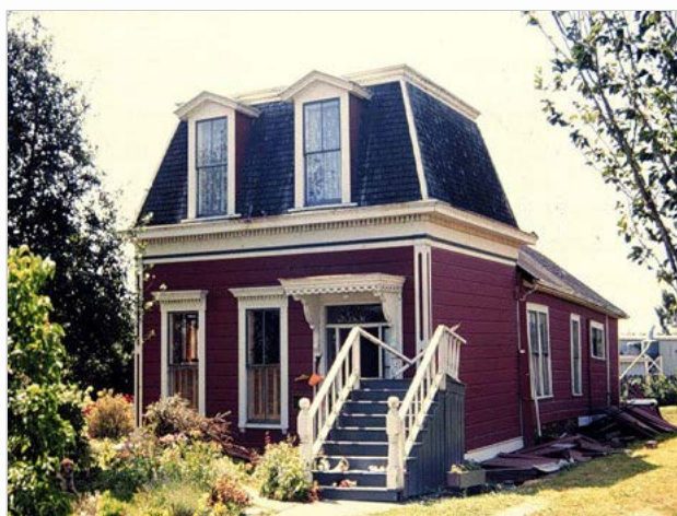
This heritage home in California dropped by half a storey in an earthquake
