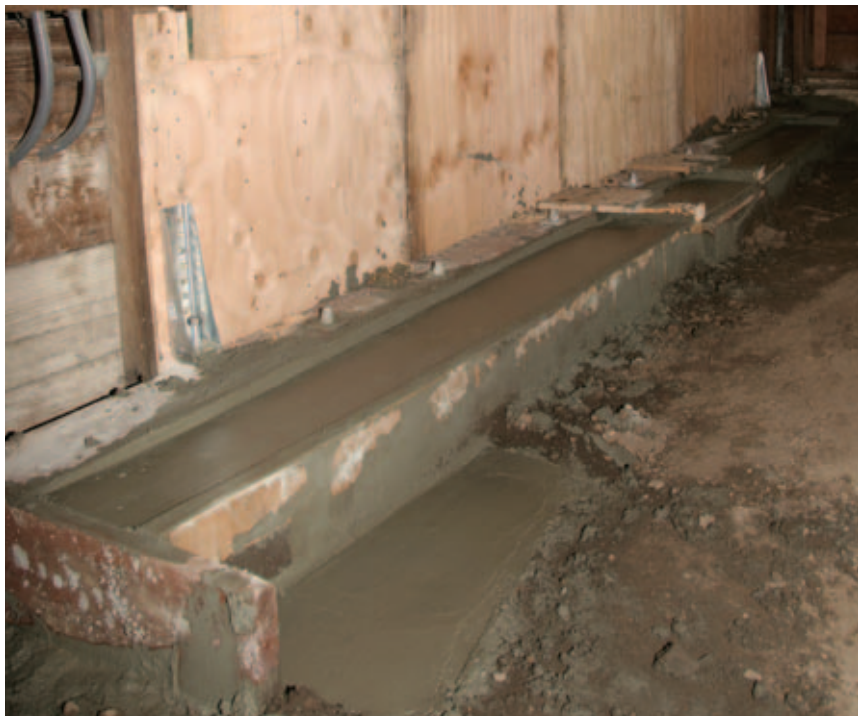
Figure 9. The foundation under this shear wall can support the vertical load but is too weak and shallow to accept hold-downs. Instead of replacing it, the author poured a new reinforced footing alongside the existing one. To tie into the new footing, the hold-downs and anchor bolts are on the interior face of the wall and attached through a “reversed” mudsill. The crew nailed the plywood to the back of the mudsill before standing it up and nailing it to the studs.
