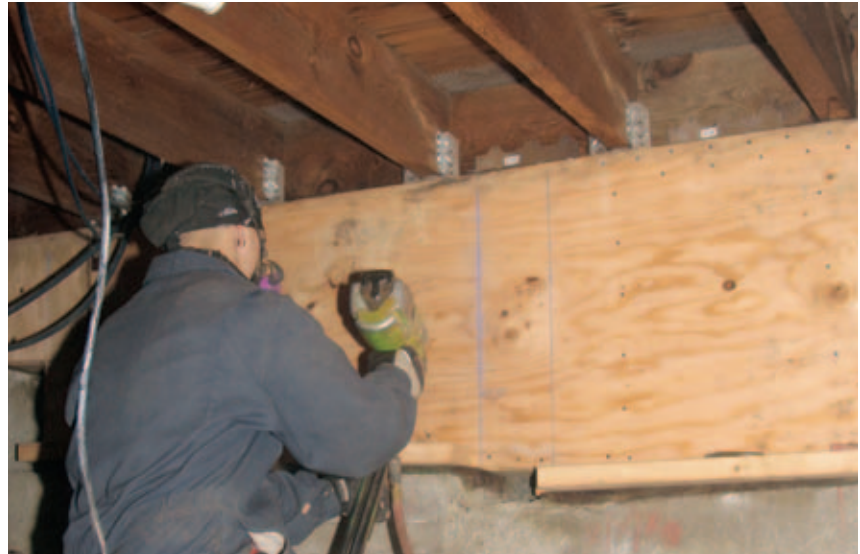
Figure 8. With the anchor bolts and framing hardware installed, this carpenter finishes the job by sheathing the cripple wall with plywood. For best results, use at least 15/32 Structural 1-grade 5-ply plywood.
