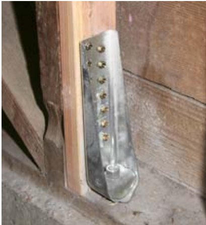
Figure 5. Now that hold-downs are installed, this wall will be sheathed with plywood and turned into a shear wall. The hardware is necessary where a wall is tall enough that overturning forces could result in uplift. It isn't needed on shorter cripple walls.
