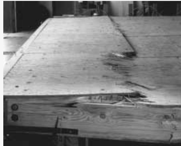
DIAPHRAGM 10 AFTER FAILURE.
