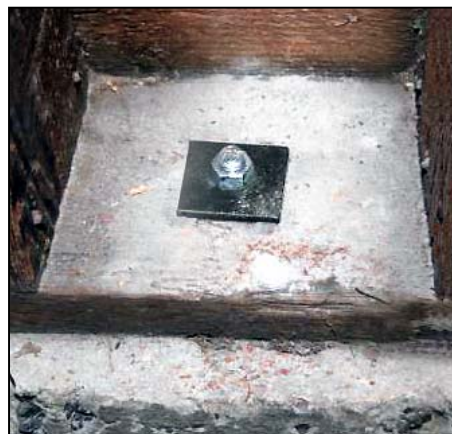
Bolt with plate washer passing through mudsill and into foundation.
