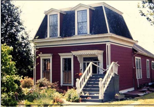
Example 1: Cripple wall failure; notice the location of the steps relative to the floor.
