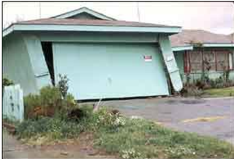
Shear walls on either side of a garage with overturning damage
