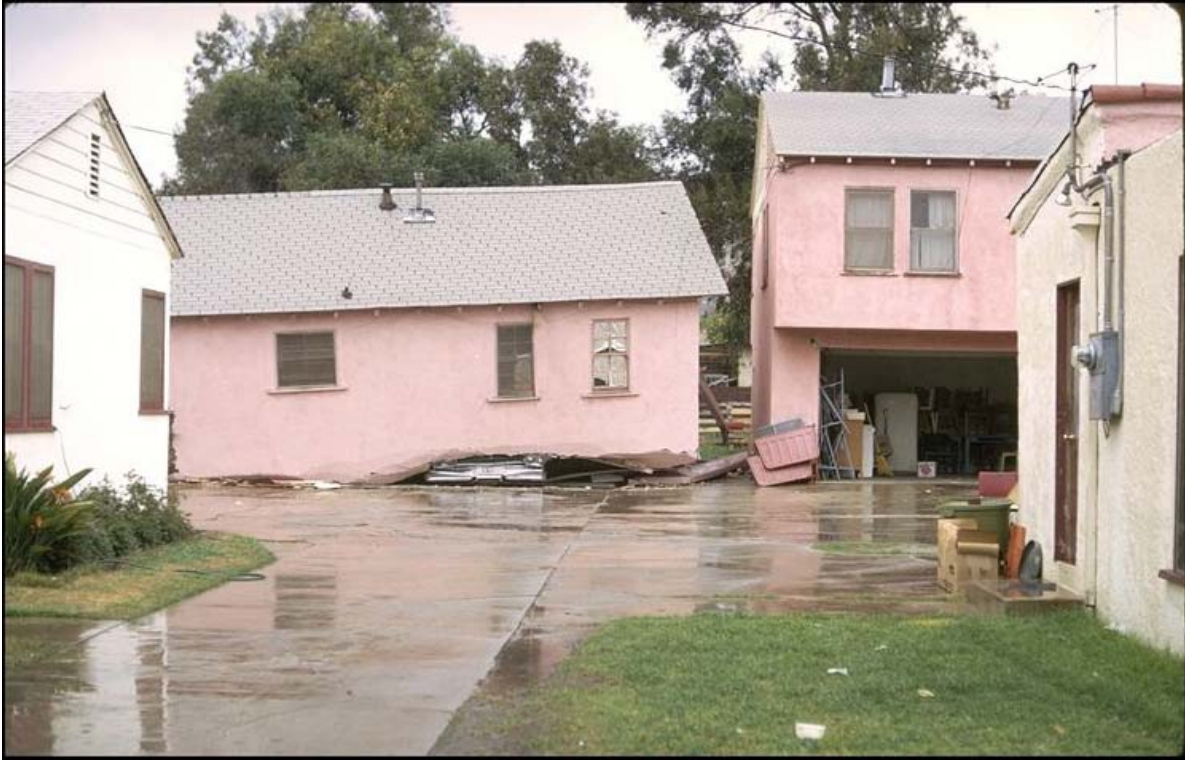
The building on the left used to be two stories. This collapse was caused by overturning of tall narrow shear walls that could not resist the earthquake forces generated by the heavy living area above a garage
