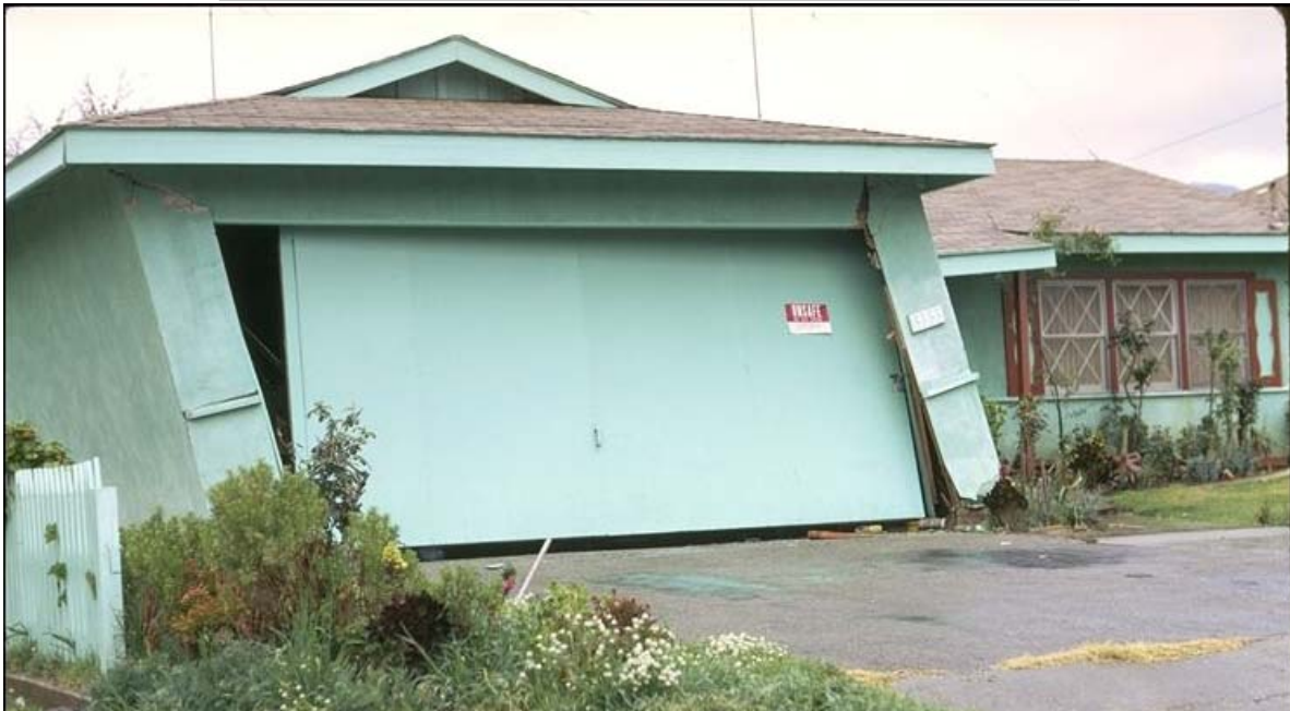
Overturning damage caused to shear walls at front of garage.
